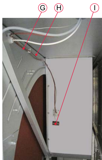
Figure 3.20 Câble PT1000 (G), câble HTCO (H), tuyau (I)
