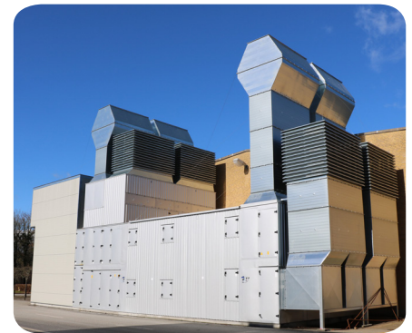
One of the two largest plants at 126,000 m 3 /h has replaced 6 smaller plants and ensured major savings.
