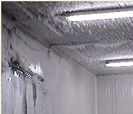
Extreme icing on the ceiling.
