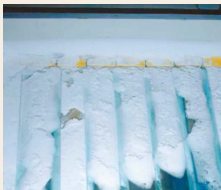
Ice build-up in the loading dock.
