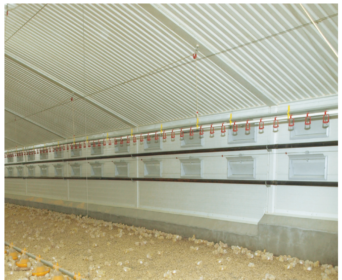
Several IW Air inlets mounted into a poultry house.
