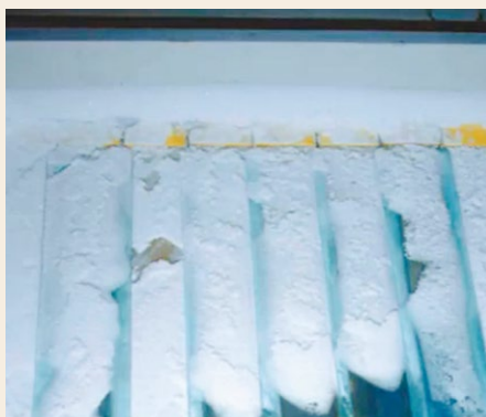
Ice build-up in the loading dock.
