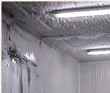
Extreme icing on the ceiling.
