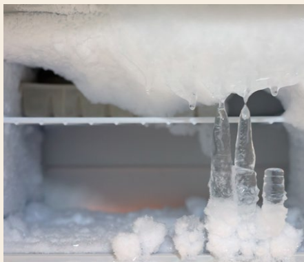
Ice forms on fixtures and equipment.
