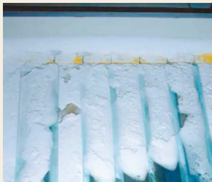
Ice build-up in the loading dock.
