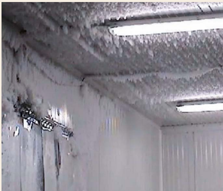
Extreme icing on the ceiling.
