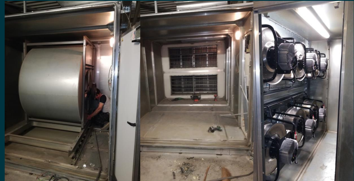
Munters helped Liège Airport modernized its passenger terminal climate control units
