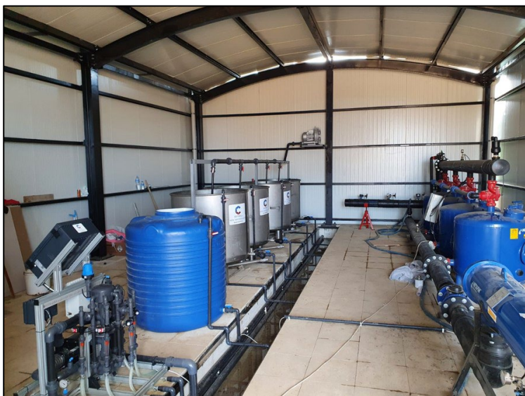
Figure 1: Green JET Unit, Installed and Running
