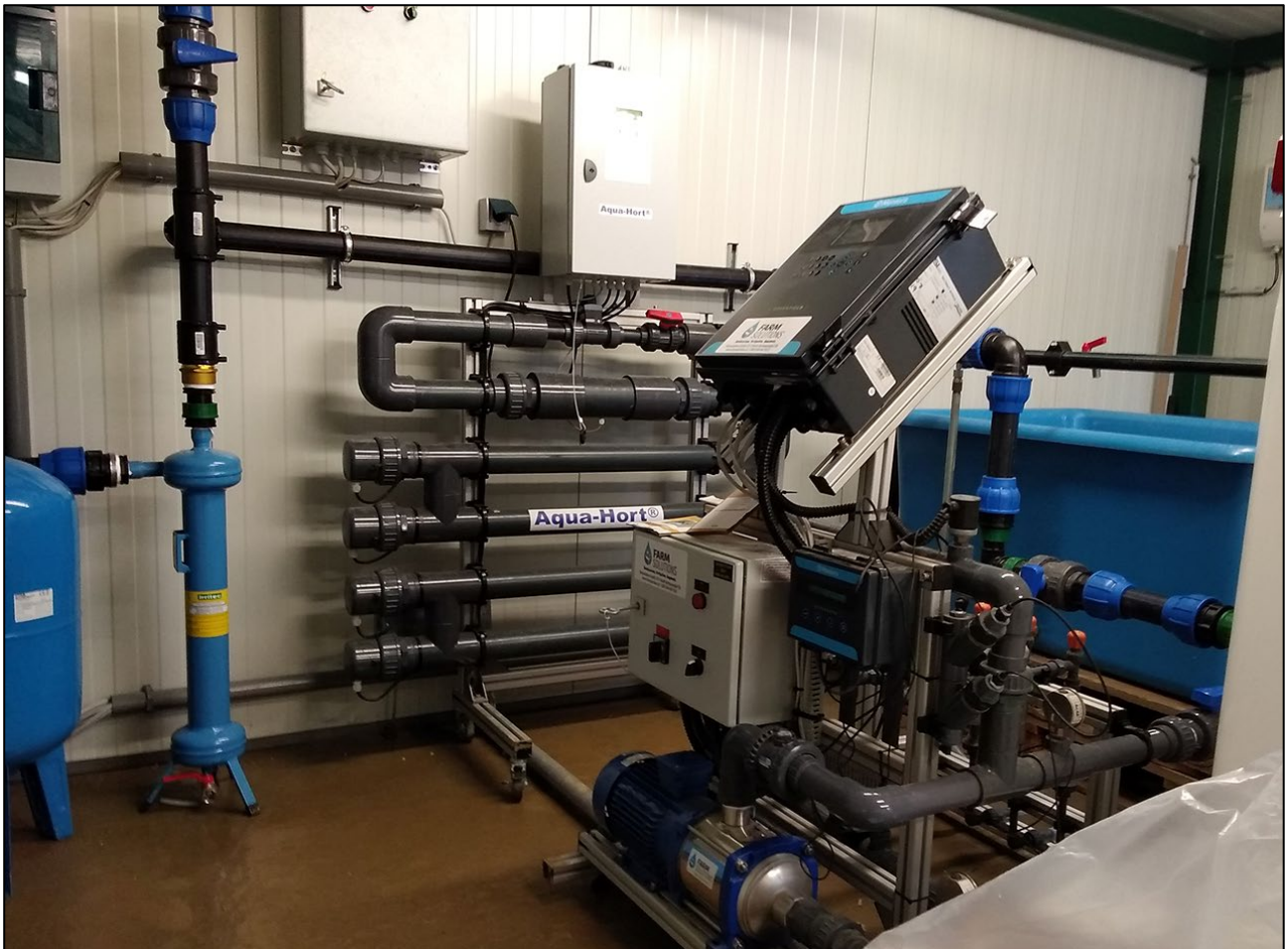
Figure 6: Green JET EC pH Unit in Place
