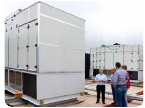
The Oasis™ 200 units are placed on the roof, directly above the server aisles.
