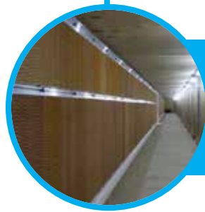
CT Cooling with CELdek
