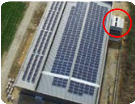
The two Oasis™ 200 units, placed next to the solar panel covered energy efficient Data Centre facility
