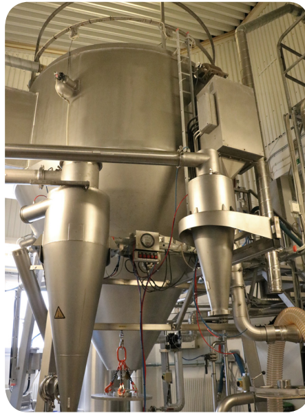
The spray tower in which 13 tons of pollen powder is produced annually by means of dry air from a Munters desiccant dehumidifier.
