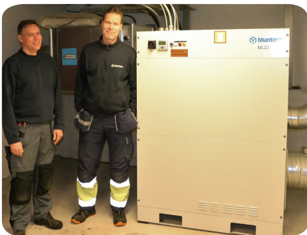
Ted Johansson and Munters service technician Roger Johansson next to the new ML23 dehumidifier.
