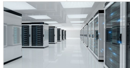
Data Center cooling solutions
